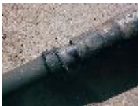
Figure 6: Shifter Linkage Weld
